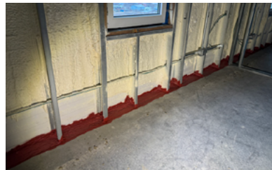
Firestopping between floors
