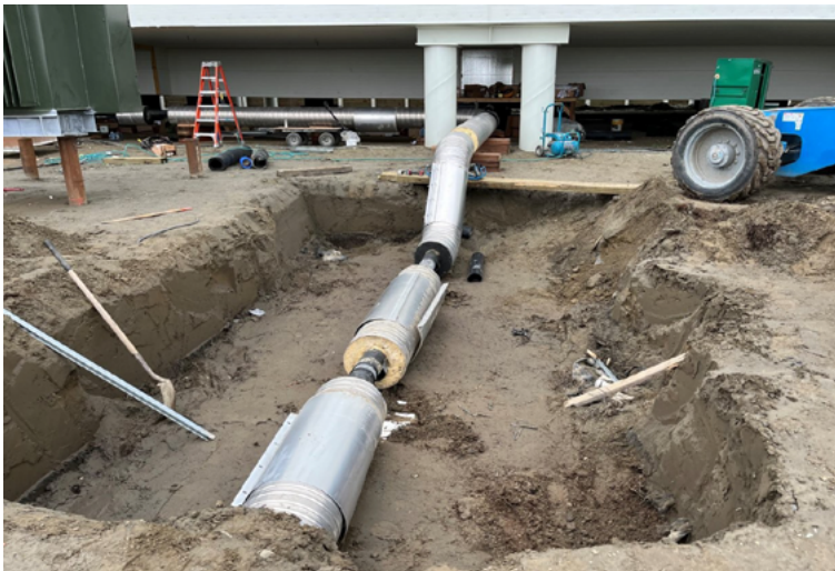
Tuntu Apartments - Arctic pipe water main to building
