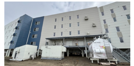
Lift station building, generator and fuel oil tank at maintenance deck
