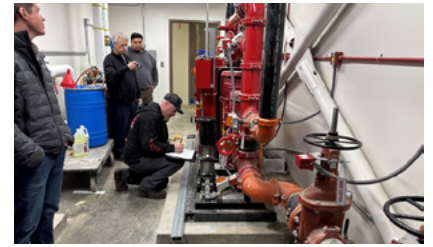
Fire pump training and testing
